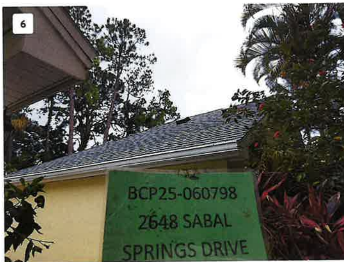
Project: 2648 Sabal Springs Dr unit 6 Date: Jul 15, 2025, 7:02 PM Creator: Lucio Roofer
